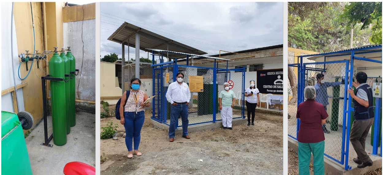
Figure 20. Health facilities with oxygen points and networks installed, or with concentrators installed / Iquitos - Lambayeque – East Lima
