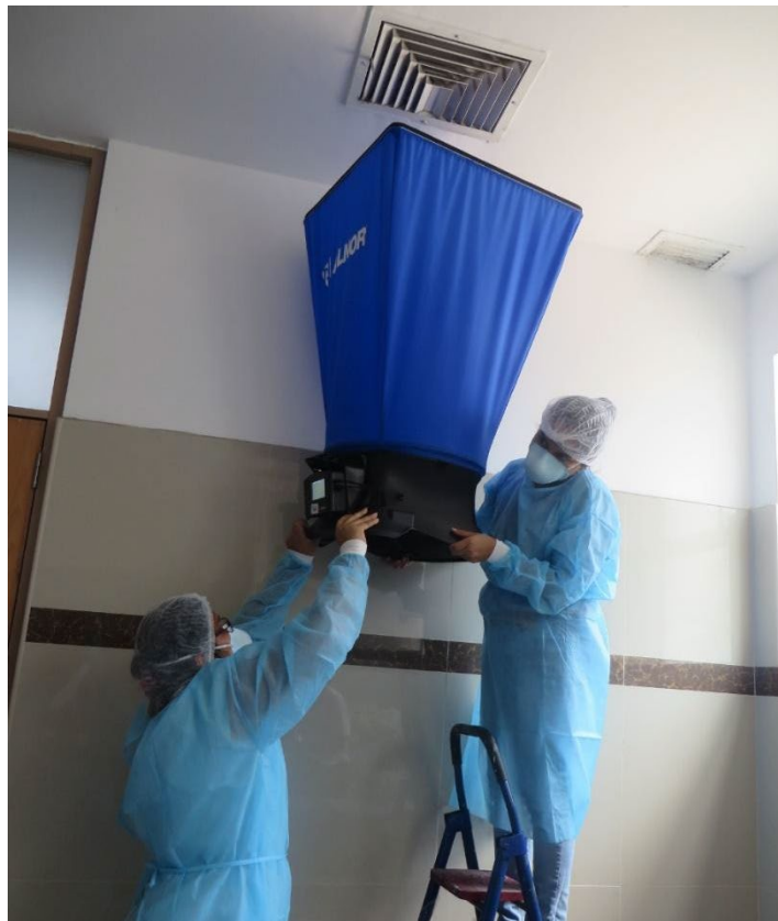
Figure 34. Measurement of air filters in hospitalization areas
