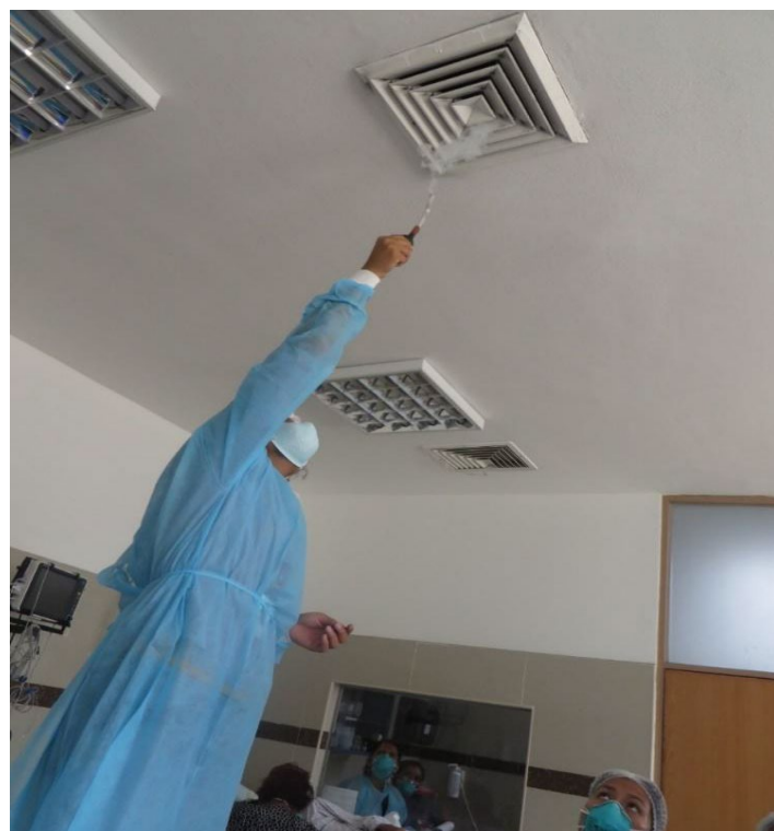
Figure 35. Air flow measurement
