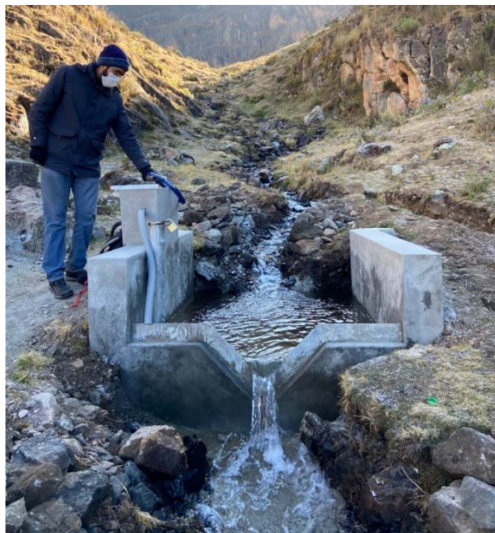
Figure 2-2. Installation of a sensor on a flow weir in Cañete
